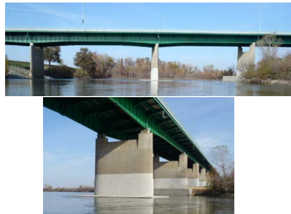
Figure 1. Multi-girder Bridge (Feather River Bridge) in Yuba City, CA. The upper photo highlights the two spans of interest for the study, span 21 (left) and span 22 (right).
