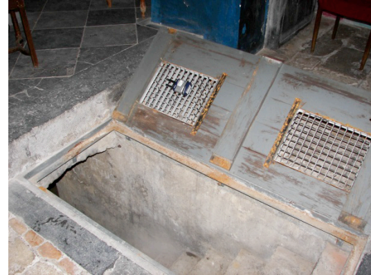
Figure 13. Crypt entrance: measurement equipment is placed on the screen of the hatch between chapel (nave) and crypt
