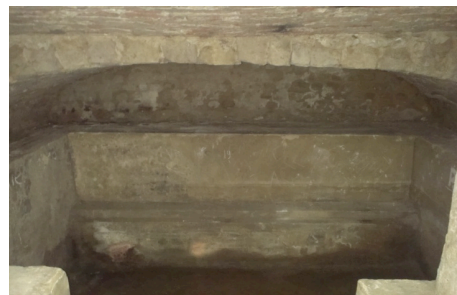
Figure 5. Entrance of the wet crypt (up) with a few centimetres of standing water (down)
